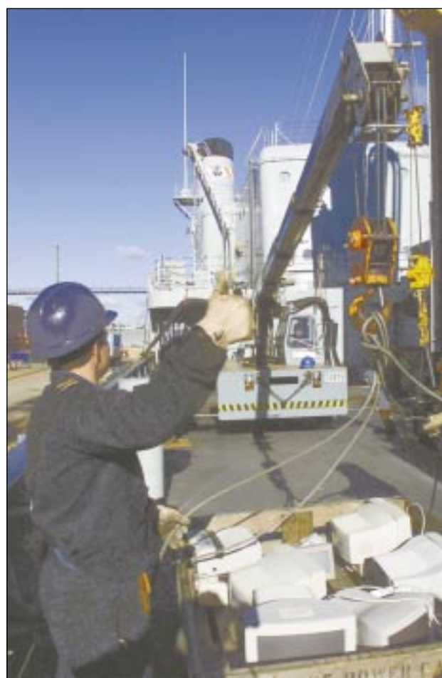
LS Grady signals thumbs up as a crane operator lowers a pallet of computer hardware.
